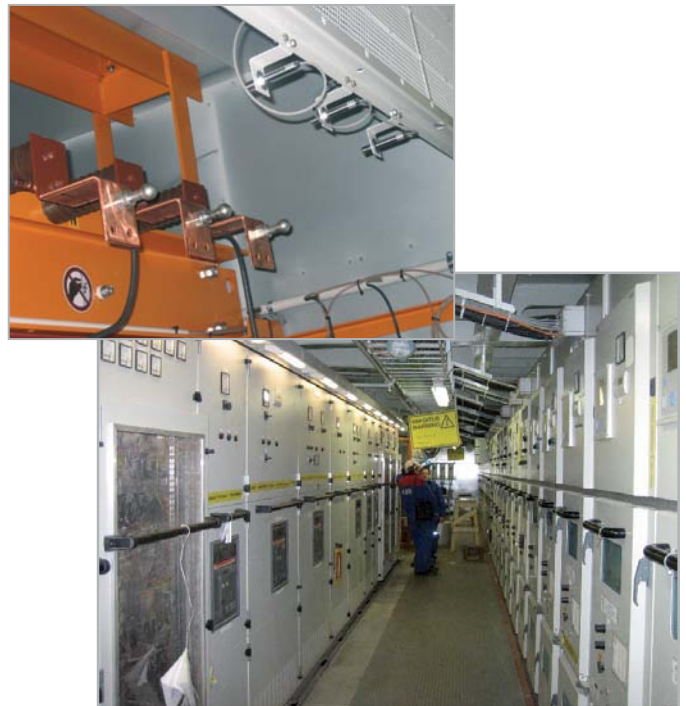
Typical monitoring locations at points of contact; Medium-voltage switchgear monitored by fixed pyrometers
